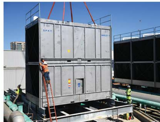
Workers install a new water-cooling tower to improve the Convention Center's HVAC systems.
