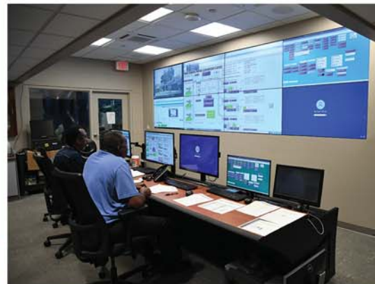
Convention Center employees helm the newly renovated HVAC Control Center.
